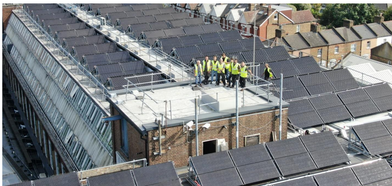
Image: Solar-PVT installation on the roof of the Ealing Campus, University of West London
